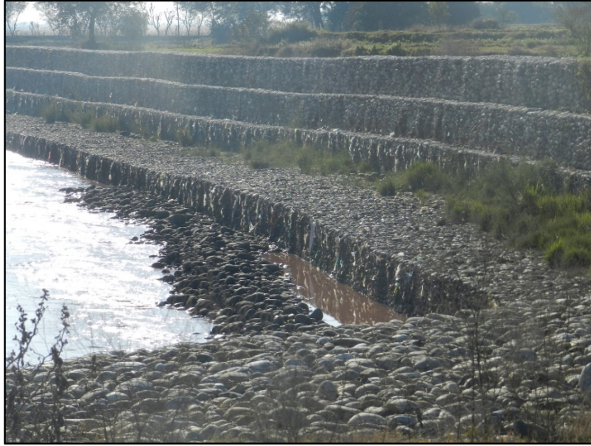
Typical bank protection works carried out by State Engineers along river Chenab, J & K
