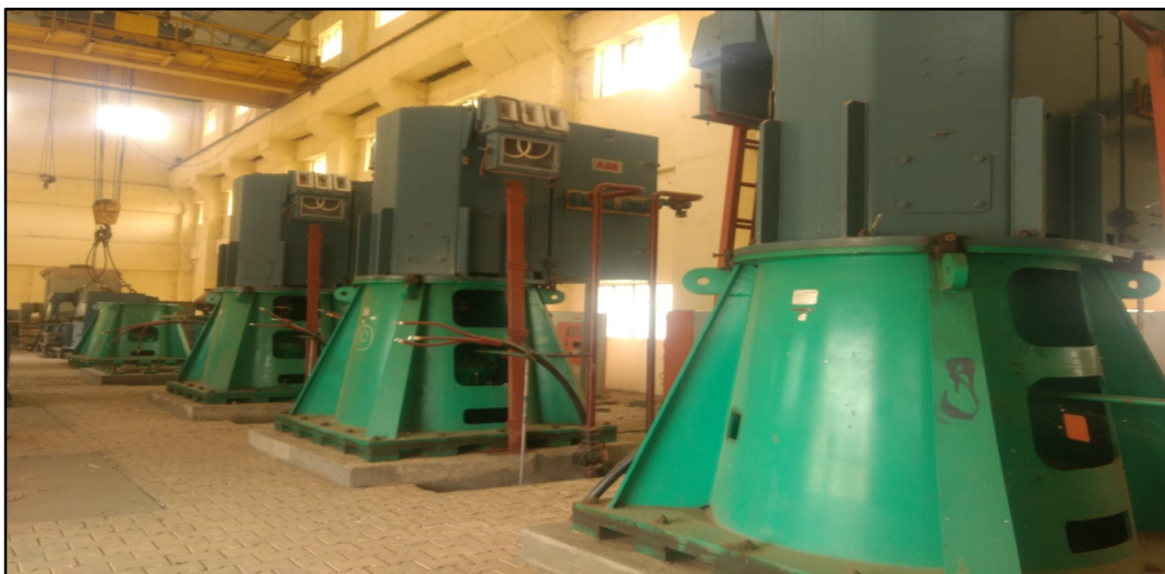
TalodhiMokasa lift irrigation scheme Pump House, Dist. Chandrapur in Maharashtra.
