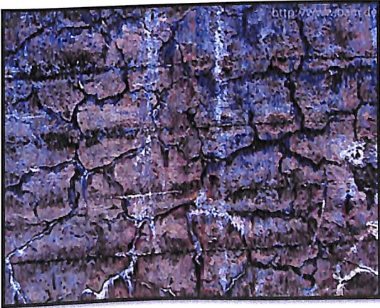
Map cracking on concrete wall
