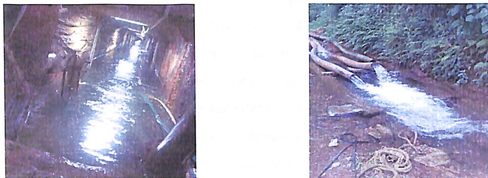
Fig. 17: Seepage in gallery & pumped out seepage
