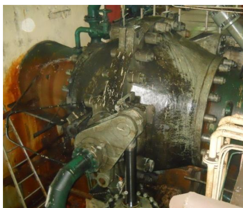
Main inlet valve of turbine at Kopili HEP
