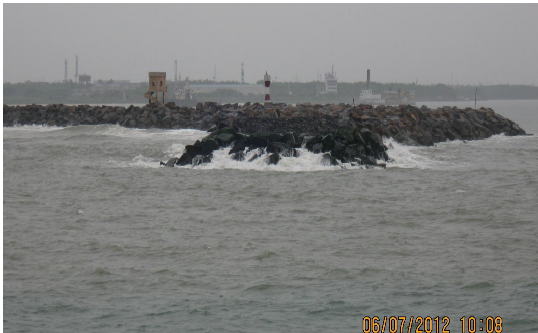
Damaged roundhead of southern breakwater
