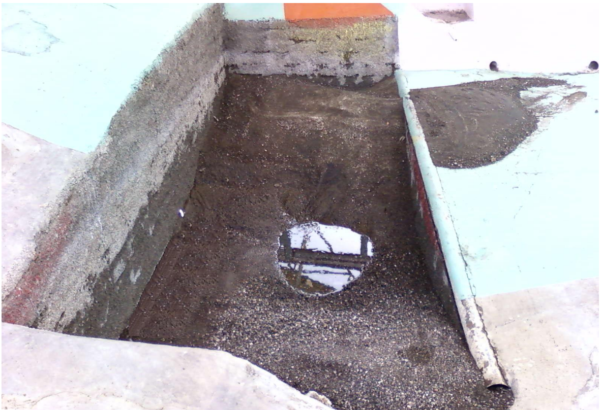
Scour downstream of spillway, Q= 1643 \text{ m}^3/\text{s} (FRL El. 1643.5 m, Gated)
