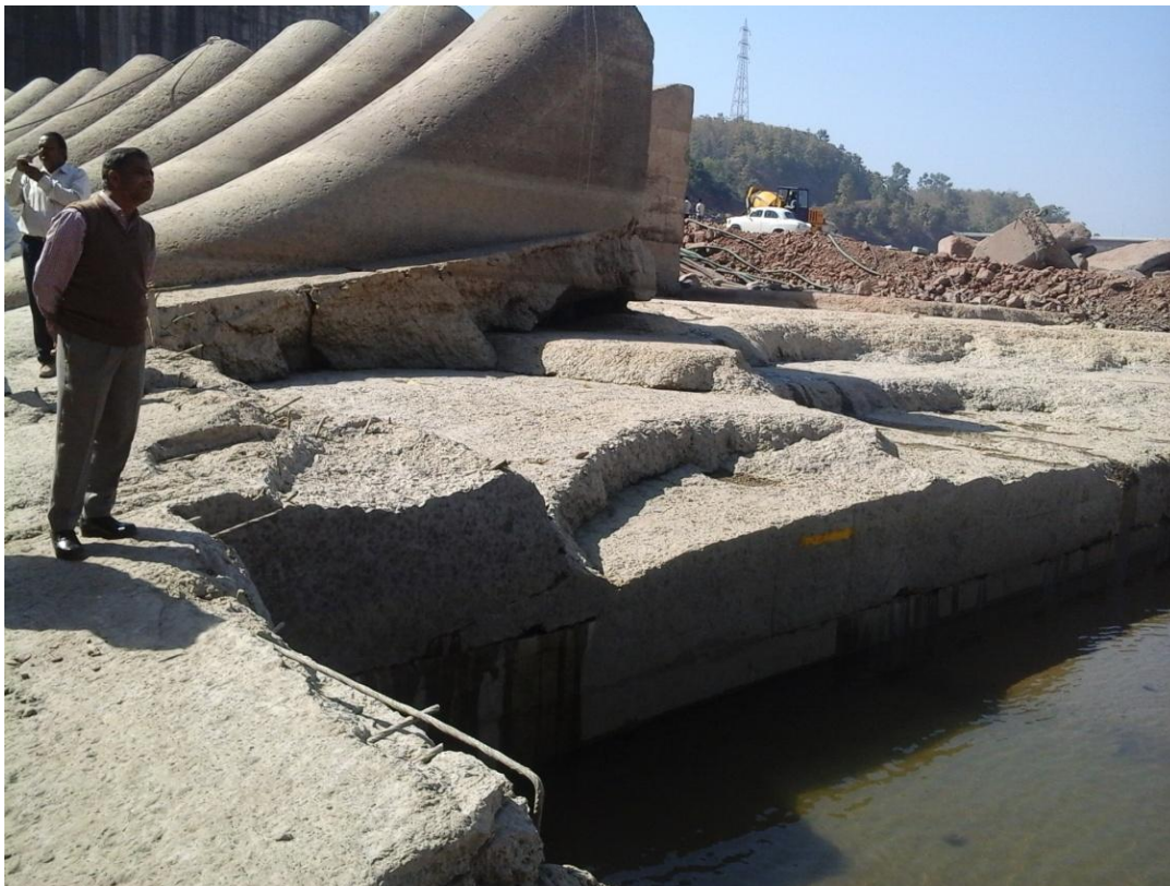
Severity of damage caused to bucket
