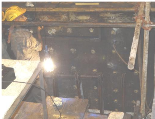
View of distressed beam
