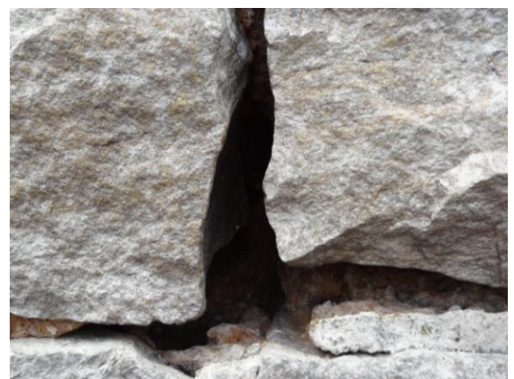
Wide openings in masonry joints
