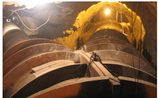
Top view of Penstock bifurcations 1 & 2
