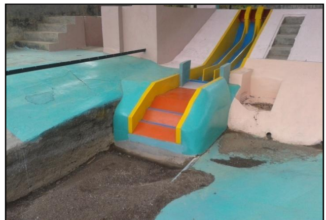
Scour downstream of spillway, Q= 675 m 3 /s (One gate in operation RWL El. 1643.5 m)
