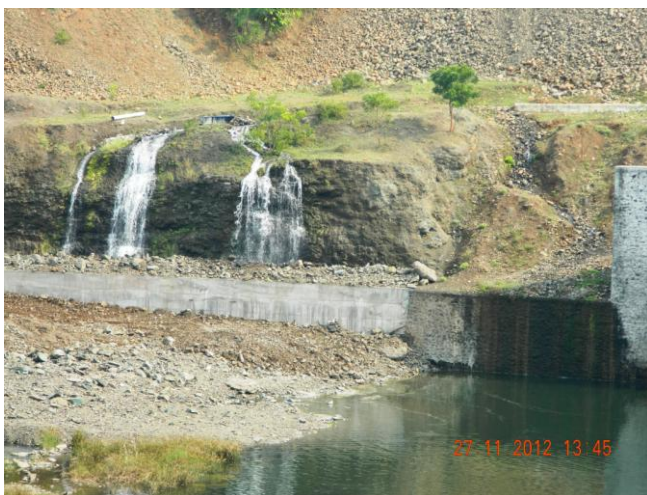
Leakage on the RH side of the dam
