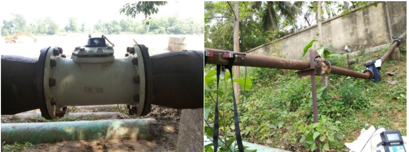
Existing Water Meters with improper installations at site
