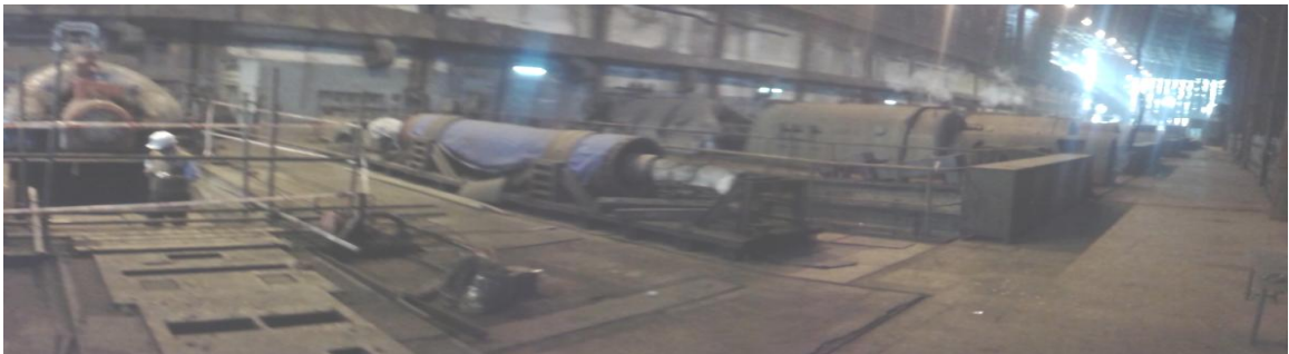
View of captive power plant - 1, R.S.P., Rourkela
