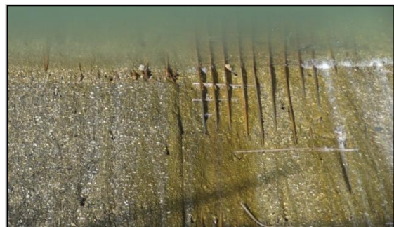
Pitting and reinforcement Exposure
