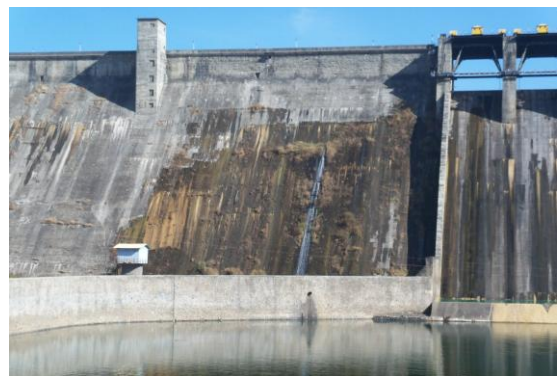
Seepage seen on d/s face
