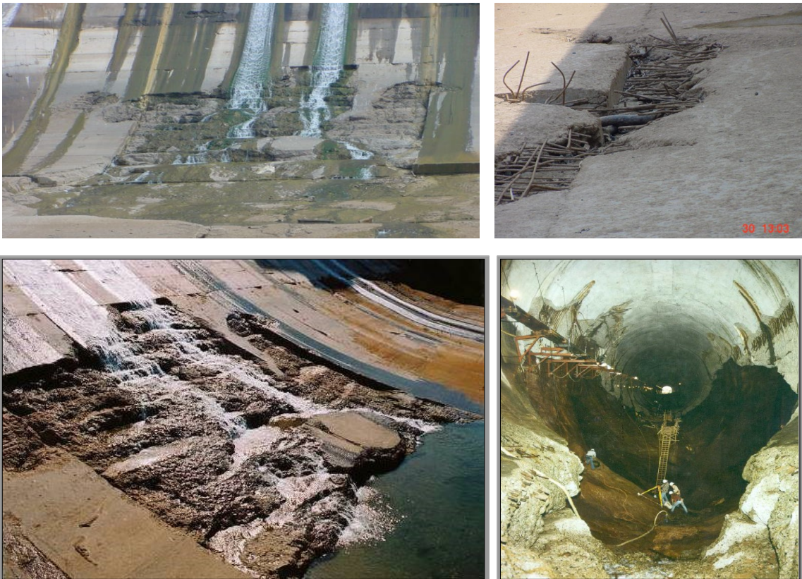
Cavitation damages on spillway surfaces
