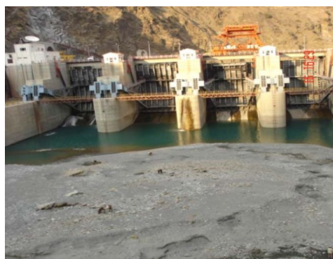
Silt deposition in the stilling basin of Chamera II Project, HP
