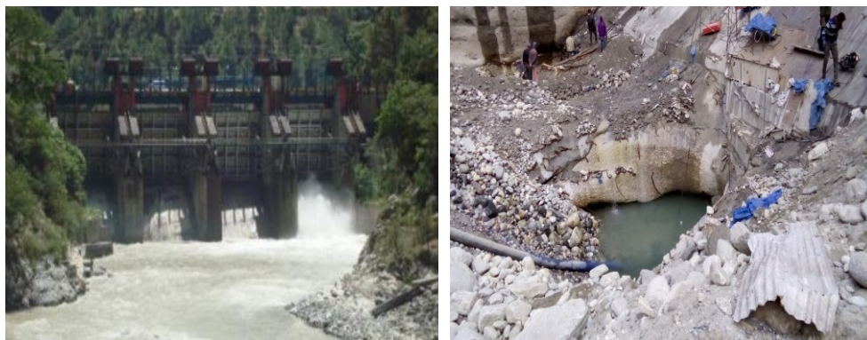
Damage to roller bucket of Maneri Bhali spillway, Uttarakhand
